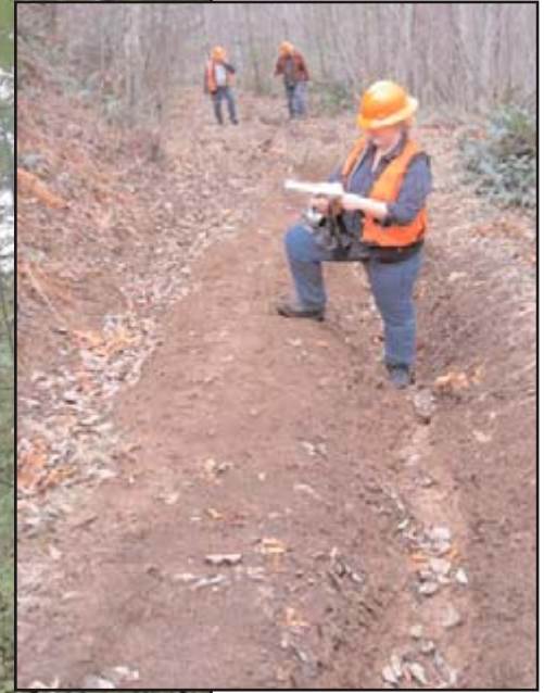
Anitra Gorham from Natural Resource Conservation Service evaluating deteriorating road condition.
